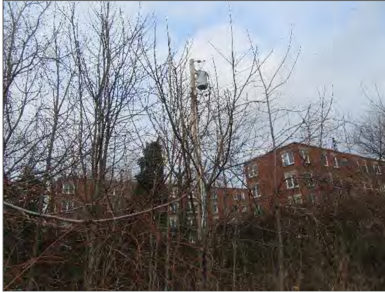
Photo 10 – Pole-mounted transformer located immediately southeast of the Phase One Property.
