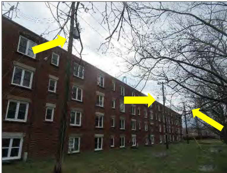
Photo 7 – General view of three pole-mounted transformers located on the central and northeast-central portion of the Phase One Property.
