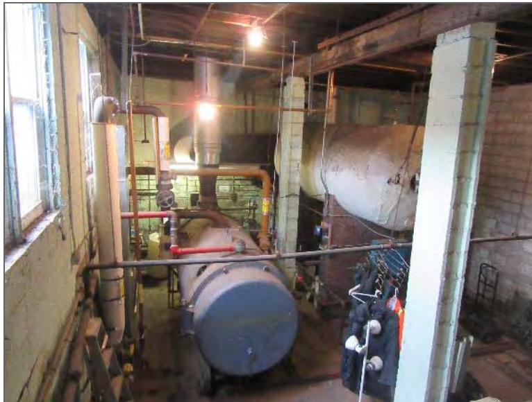
Photo 9 – Representative view of the boiler room located within Site Building C.
